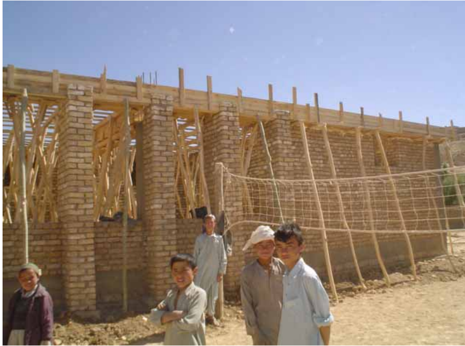
A school building under construction in Roy Do Aab District, Samangan Province.
